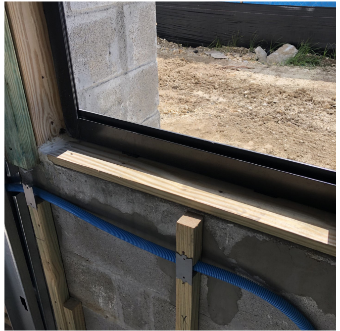
A window installation (not wrapped) resting on bare bucks will fail pressure testing 99% of the time.
